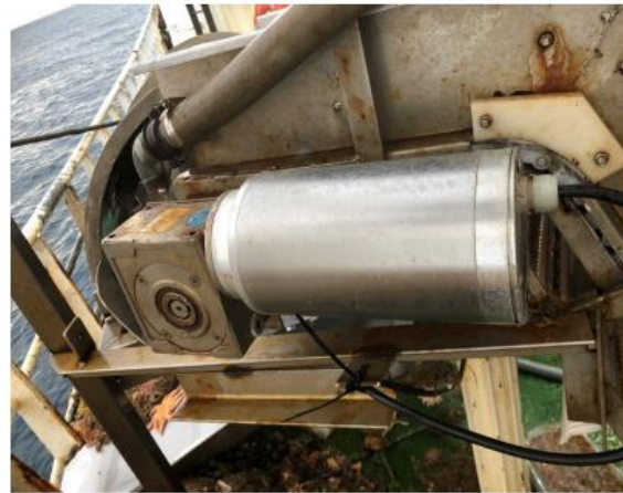
HCW motor after 2 years working in salt environment
